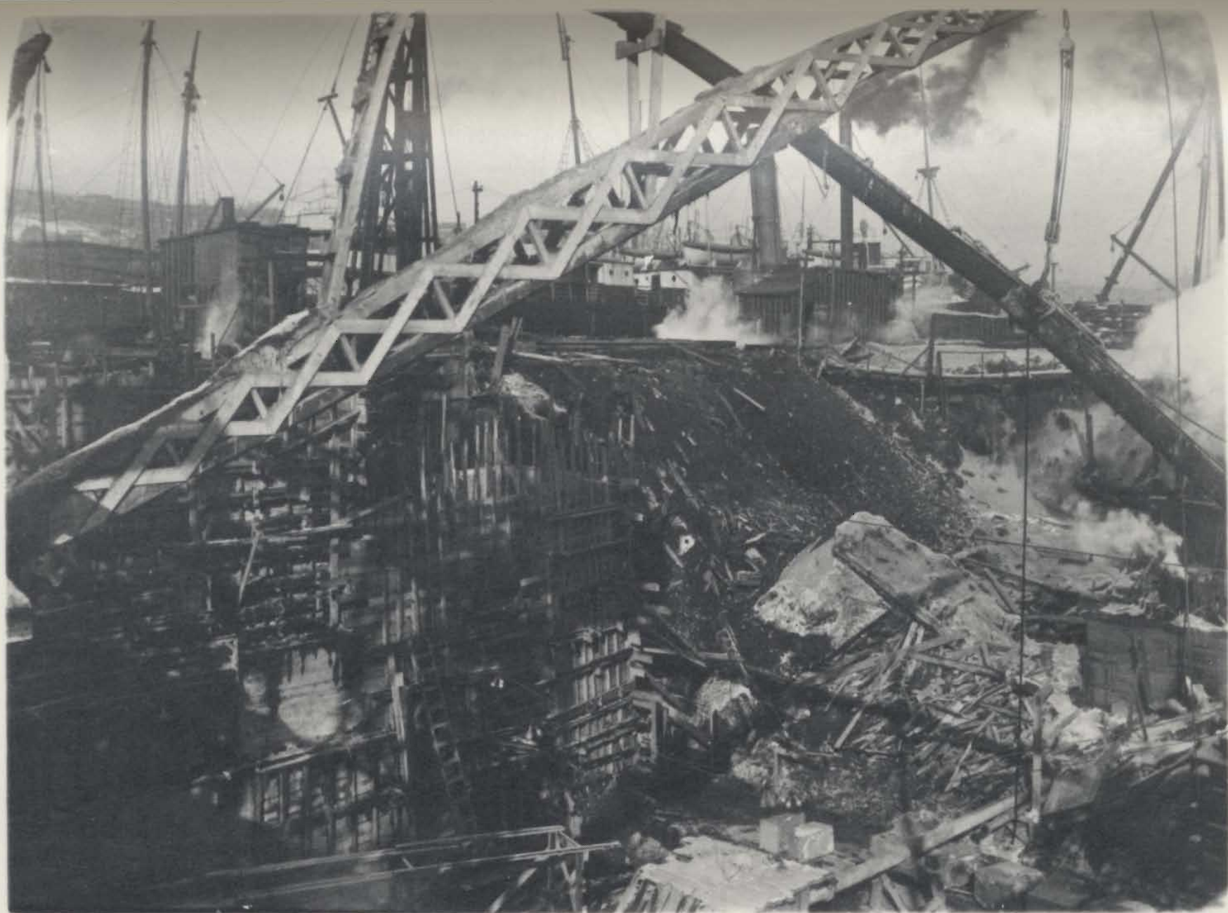
Figure 31. The St. John's Dry Dock shown here under reconstruction by the Reid Newfoundland Company which acquired the Dry Dock from the Government in the 1898 agreement. Immediately west of the Dry Dock a new station house and marshalling yards as well as machine shops to service the railway, the coastal boat fleet and the Dry Dock were built on land reclaimed from the West End of St. John's Harbour.
