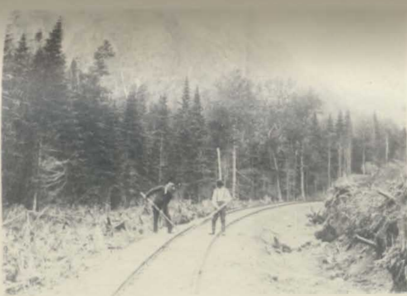
Figure 23. Section men working on the railway near Humber Mouth shortly after the completion of the railway. This short section of track was eventually moved back several hundred yards from the Humber River to make way for a highway which had to share the same route with the railway through a narrow gorge of the Humber River.
