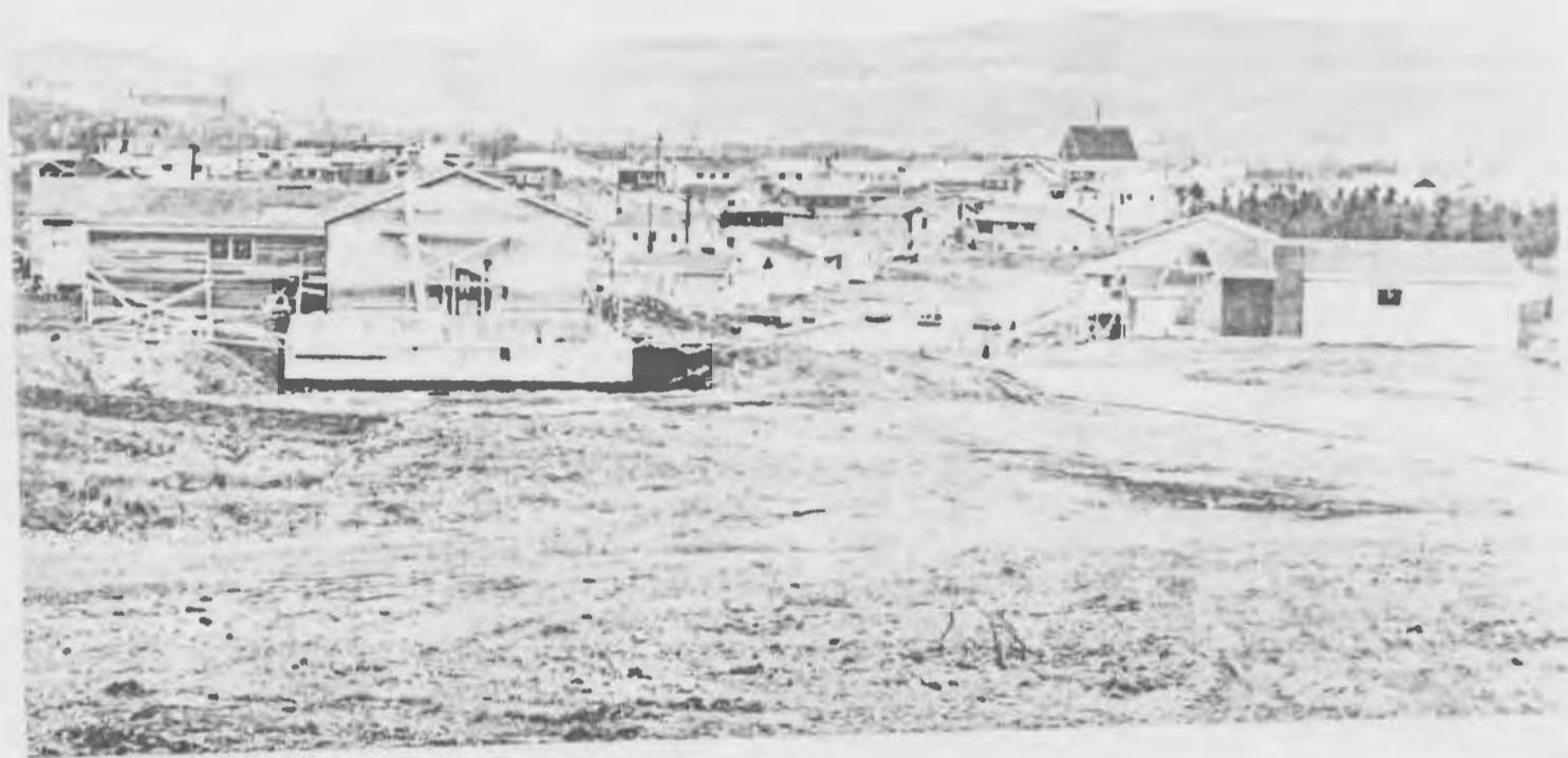
Homes Under Construction In The Northeast Land Development Area. Can You See Any Examples Of The New Contrasting And Blending With The Old.
