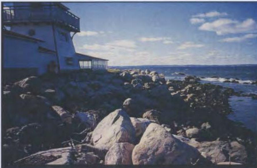
Plate 9.1: This building, adjacent to the Foxtrap Marina (segment 7866 – 7947 m), is located within the 30 m development setback and is less than five metres from the bluff edge. Although the placement of riprap will halt erosion processes, the site can still be impacted by storm waves.
