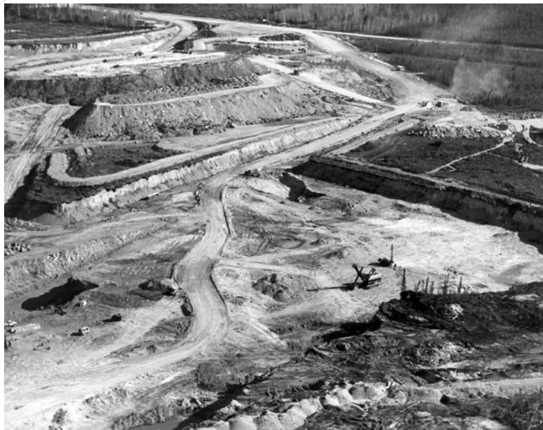
Fig. 4: Aerial view of the O.42 pit area. Pine Point, April 28, 1965. Credit: Cominco/NWT Archives/N-1987-021-0056
