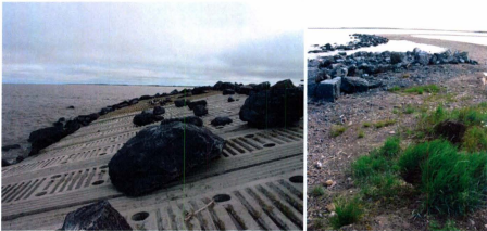
Figure 5.9 (left): Rip-rap shore protection installed in 1998, North Spit (west side). Note armourstone ‘mobility’.
