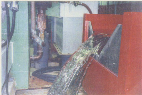
Figure 5-16 Photograph of the V-notch weir
