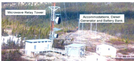
Figure 3.1: A photograph of Bell-Aliant's telecommunication site at Mulligan, Labrador
