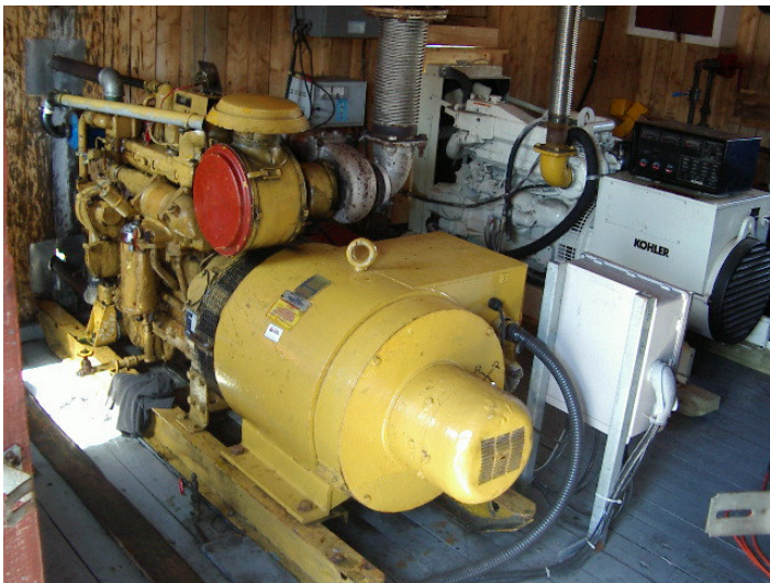
Figure 4: Battle Harbour diesel generator
