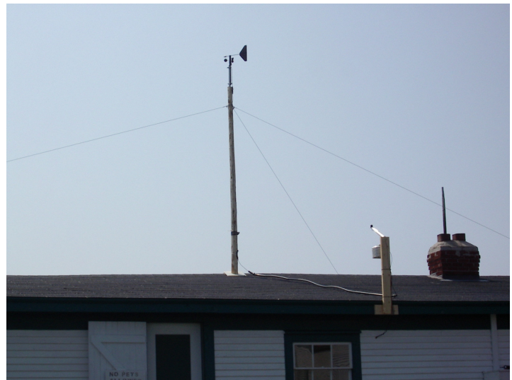
Figure 5: Installed wind equipment at Battle Harbour
