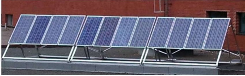
Figure 4-10 MUN ECE laboratory PV installation.
