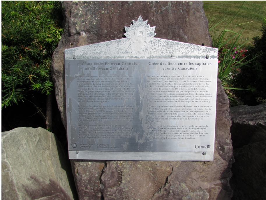
Figure 5.8 Image of the Building Links/Confederation Monument in Bowring Park. Looking at the plaque you can see it is in rough shape and needs to be redone. Emlyn Tuck (2023).
