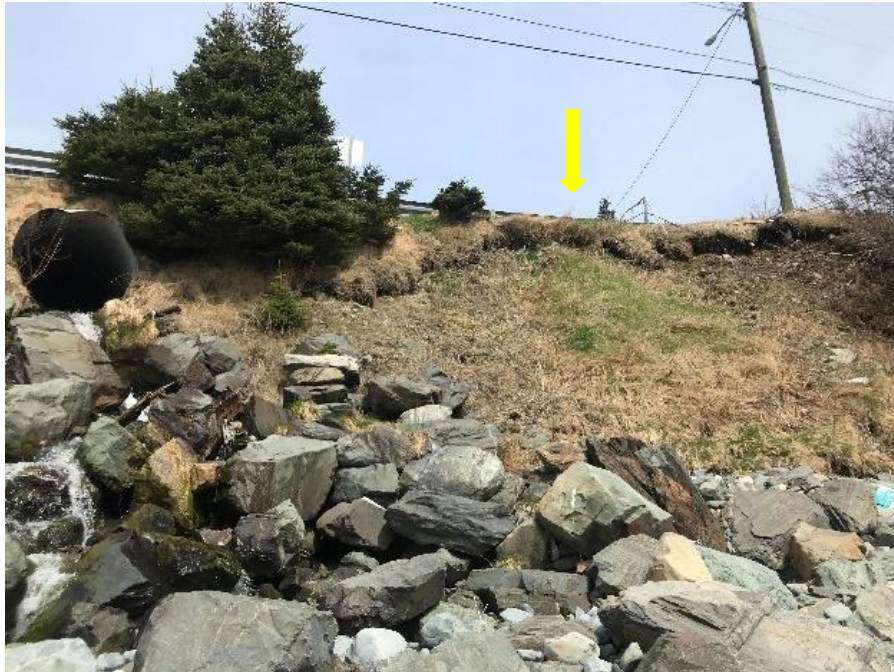
Figure 2-11) Lack of coherence in the Quaternary cover is depicted, as shown by the yellow arrow. The culvert opening appears on the left. Left and bottom: boulders (rip rap) have been brought there to stabilize the road. Photo taken from the beach, facing northeast.
