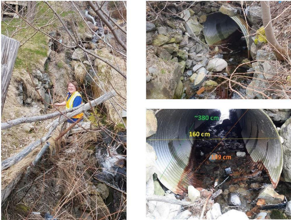
Figure 2-4) Left: The boulder-strewn creek north of the Bread and Cheese culvert. Photo taken from the road, looking north. Right: The north end of the culvert, taken from the west bank of the creek (top), and from the creek bed looking south (bottom). (22 April 2021)
