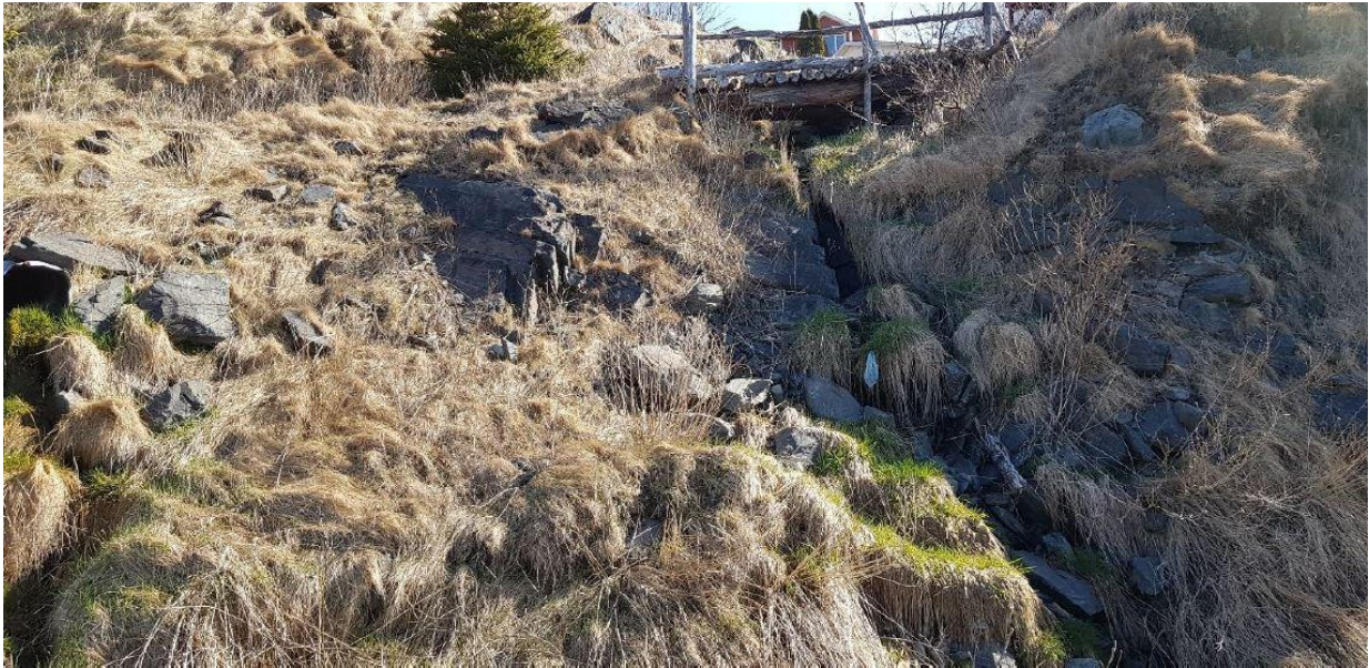
Figure 2-24) Vegetated sediment containing many angular boulders, near a fourth culvert to the southeast of the survey area (~ UTM 363300 E, 5241850 N). 21 April 2022.
