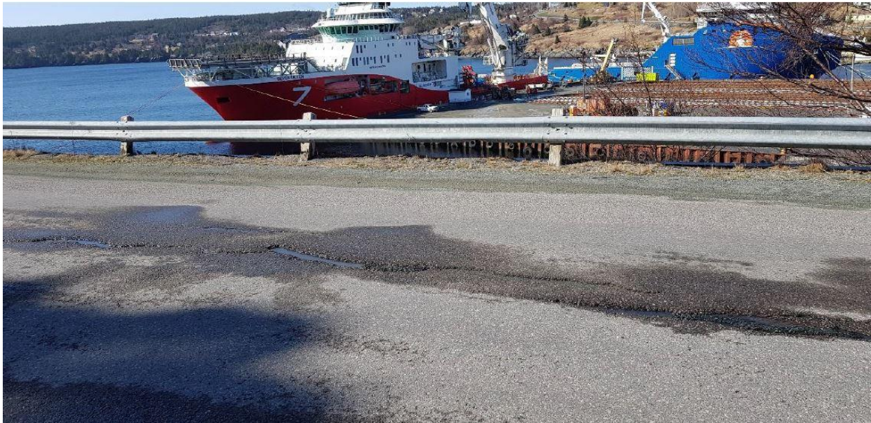
Figure 2-25) A crack in the pavement is another indication of shoreward motion of the land in this location. UTM 363253E, 524900 N. Photo taken looking south.
