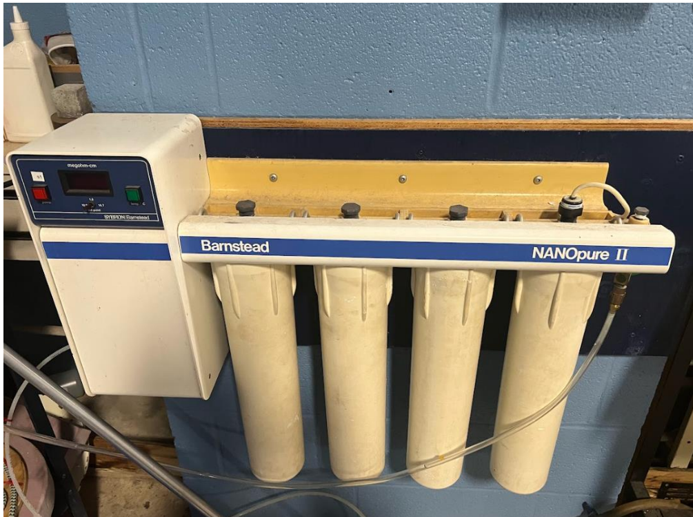
Figure 29 – Water deionization system.
