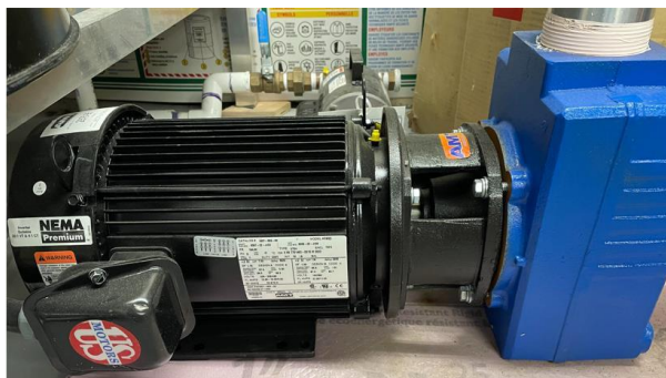
Figure 3.2: Centrifugal pump coupled to the recirculation flume.
