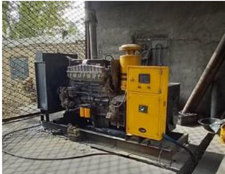
Figure 24: Primary diesel generator which is used in this site
