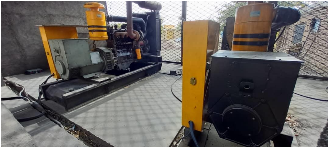
Figure 16: Current operating generators
