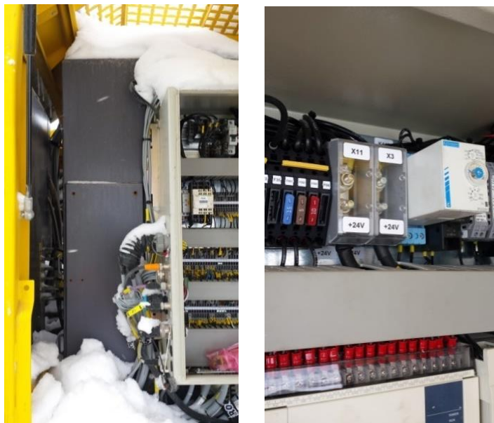
Figure 3-12 Steel mount for DAQ system 24V supply inside A1 panel
