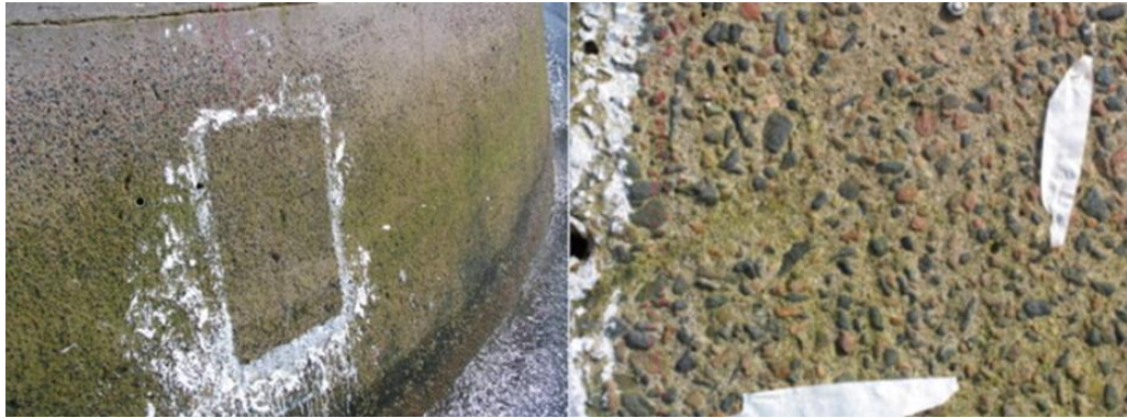
Fig. 1-1 Effect of interacting with moving ice on the concrete of pier 23 of the Confederation Bridge, from Newhook and McGinn (Newhook and McGinn 2007).
