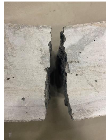
(2) Enlargement of the produced crack
