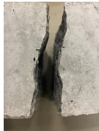
(2) Enlargement of the produced crack
