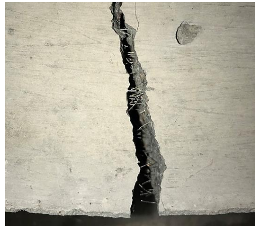
(2) Enlargement of the produced crack
