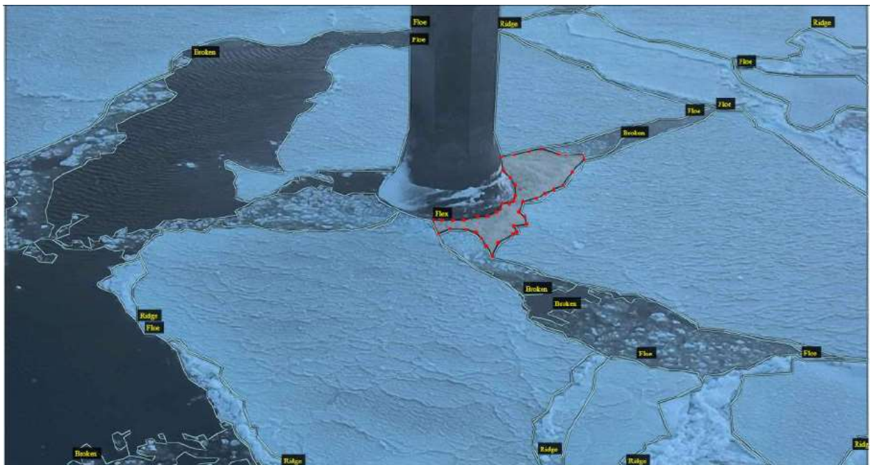
Figure A6. Example of flexural ice failure on the pier cone (gray areas outlined in red) from Figure A2.
