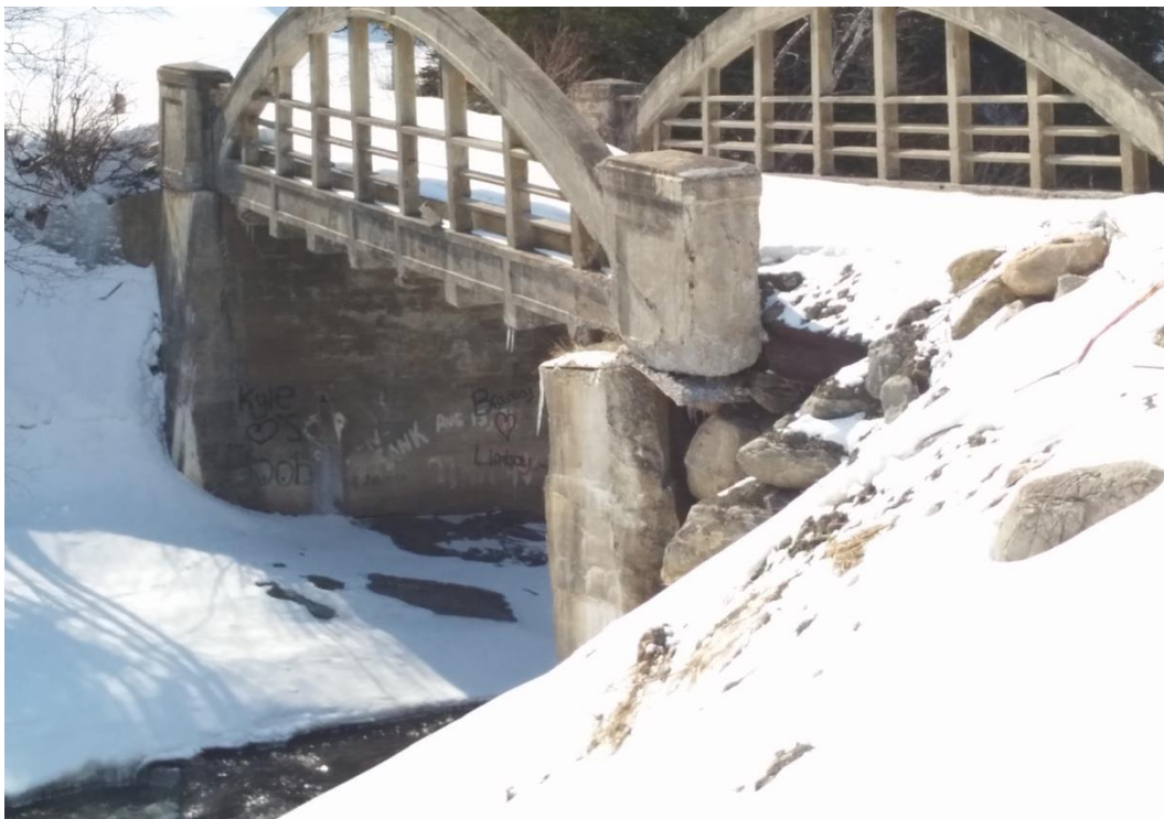
Figure 20: Damage to a secondary bridge in GBS from gradual deterioration and flooding in January 2018.
