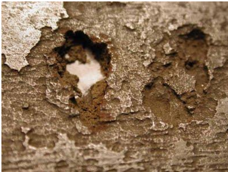
Figure 4.1: MIC pits in a steel tank substrate (Stephan, n.d.)
