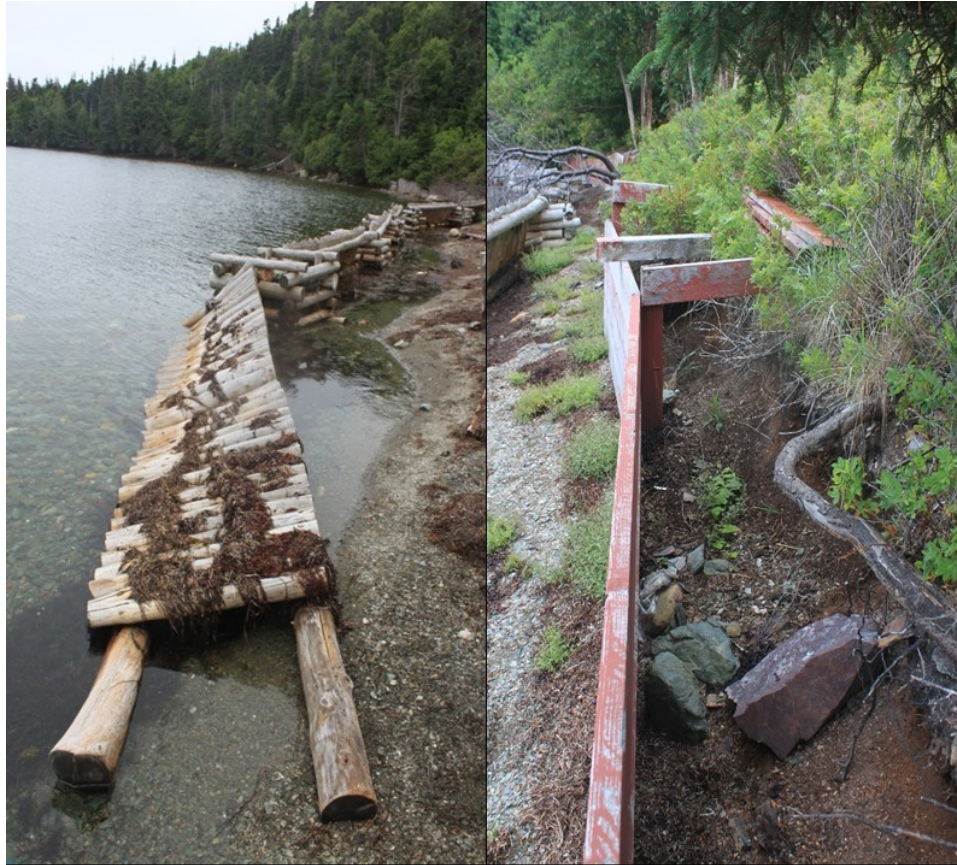
Figure 2.3: On the left: Image of first breakwater constructed to protect the Beaches site in 1995 and 1998; On the right: the second breakwater constructed to protect the site; Note: In both of these photos, it is evident that the protective measures at the site are not able to stop erosion completely.
