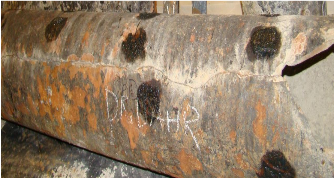
Figure 3-1: Pipe sample exhumed from the city of Mount Pearl
