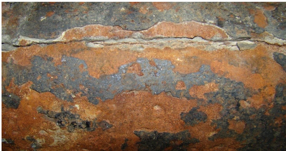
Figure 3-2: Deterioration on pipe wall
