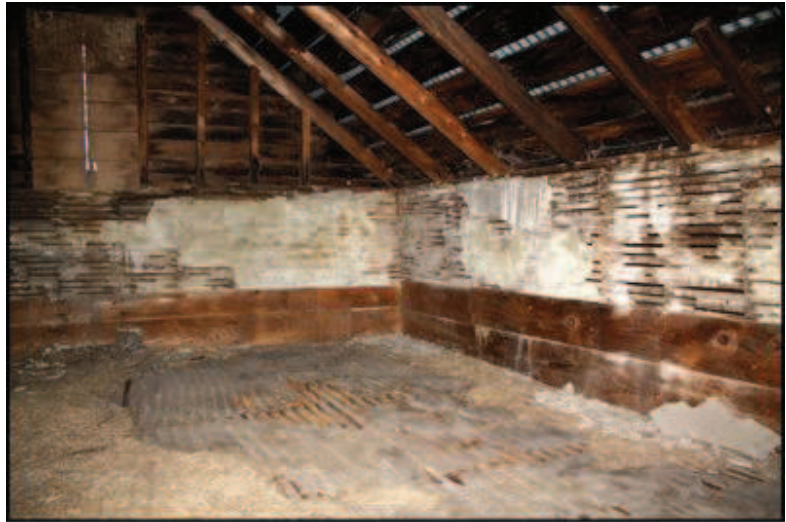
FIGURE 3.5 DRYING ROOM, SONDERGAARD HOP HOUSE, TOWN OF DECATUR.
